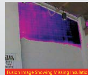
Fusion Image Showing Missing Insulation
