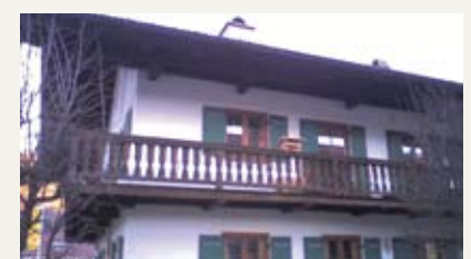
Bad insulation above balcony window
